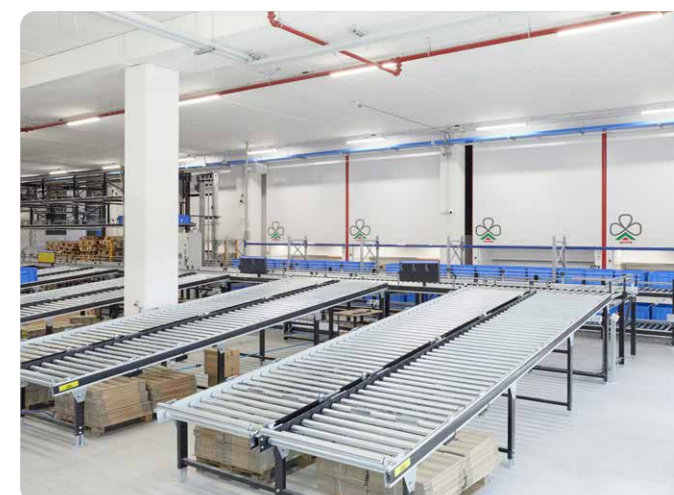
CONVEYOR BELTS AND ROLLER UNITS
